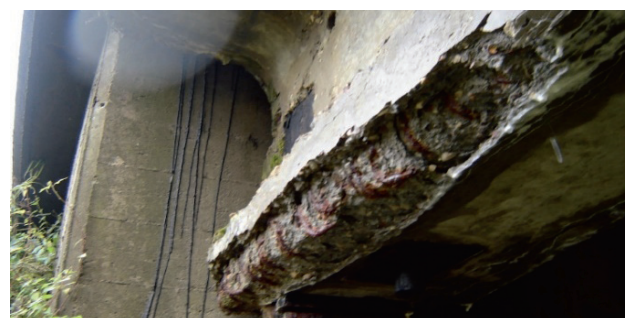
Fig. 3. Destruction of concrete protective layer and intense corrosion of primary reinforcement steel
