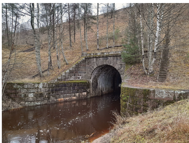
Fig. 8. Modern view of the embankment of the former railway bypass and culvert arch over the Verebya River. Photo by Dmitry Ratnikov. 2023 10
