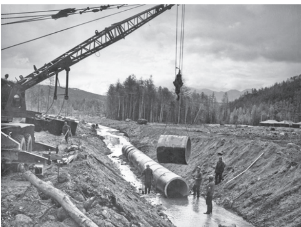
LIIZhT students building a drainage collector for the east portal of the Severomuysky Tunnel. The Buryat section of the BAM. 1977. (Photo by S.F. Spiridonov, collection of A.V. Kabanov. Science and Technology Library. PGUPS)
