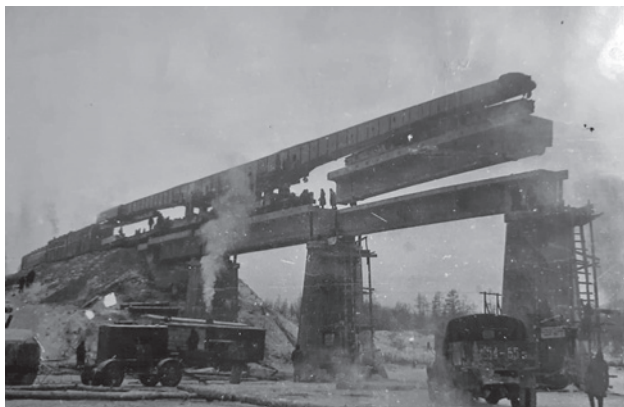
Military railway workers are replacing temporary spans with permanent ones on the river between 70 km and 90 km from Tynda. Early 1980s. (Photo from the collection of N.S. Rogalev. Science and Technology Library (NTB) of PGUPS)
