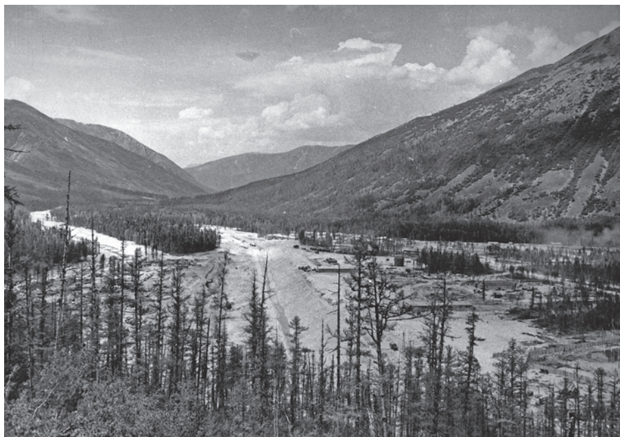
Buryat section of the BAM line. 1977. (Photo by S.F. Spiridonov. Science and Technology Library (NTB) of PGUPS)
