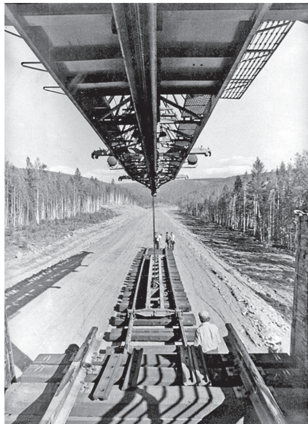
Track laying on the central section of the BAM. 1970s. (Science and Technology Library (NTB) of PGUPS)
